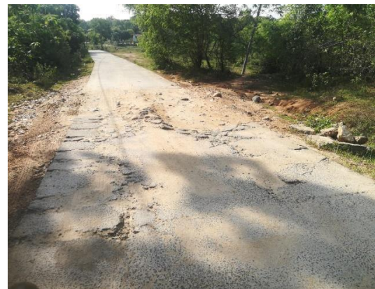
Photo.2: Destruction of roads due to carry overloaded vehicles at village
